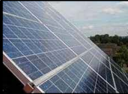
SOLAR WATER HEATING
